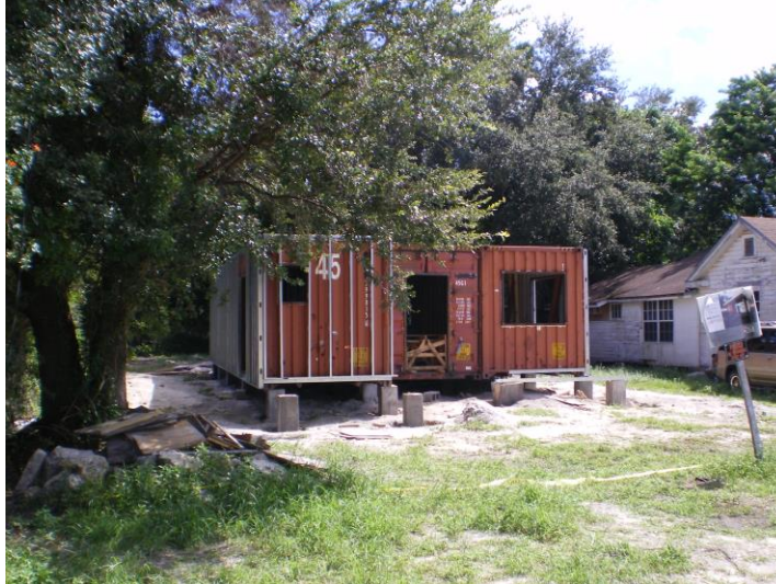
Project Name: Innovation build house with waste container and green house Project Location: Miami, Florida Design, Drawings, Calculation CE, SE, MEP, inspection, and Construction Administration by: Bijan Abidian DATE: 2014-15
