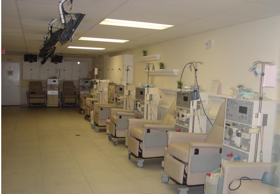
Project Name: Dialysis Center Facilities Project Location: Daytona Beach, Orlando, Boca Raton Design, Drawings, & Calculation CE, AE, SE, & MEP by: Bijan Abidian DATE: 2015-2017
